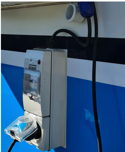
Standby 240V charger
