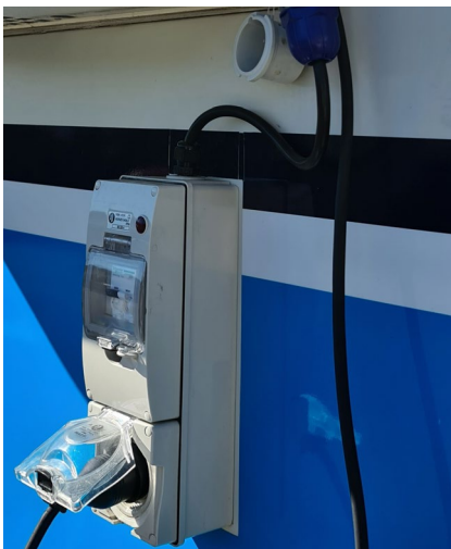
Standby 240V Refrigeration
